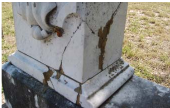
Figure 4-45. This broken marble stone was poorly repaired with epoxy. JMA, 2009.
