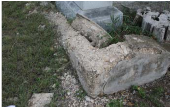
Figure 5-46. This concrete curb shows damage, likely from a rider mower. JMA, 2009.
