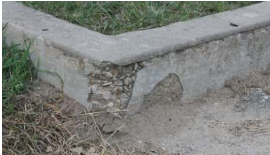
Figure 5-45. This concrete curb is disintegrating. This two-pour technique may have been executed incorrectly. JMA, 2009.
