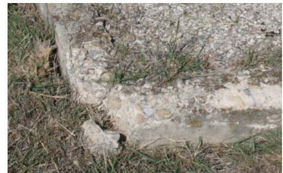
Figure 4-31. Curb failure from disaggregation combined with careless maintenance practices. JMA, 2009.
