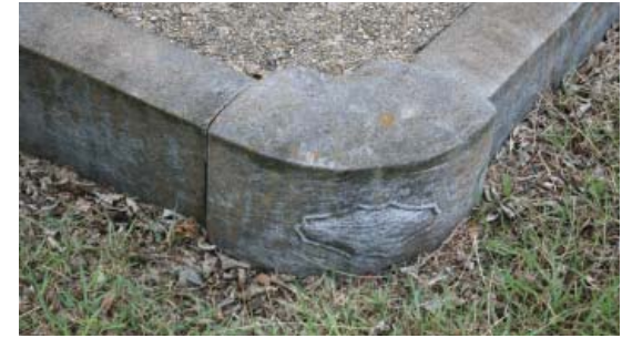
Figure 5-41. Grey granite curb with pier displaying Classical ornamentation. Note damage by weed trimmers at corner. JMA, 2009.
