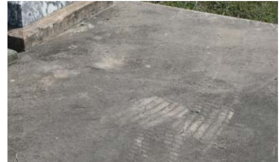
Figure 4-29. Tire tracks from a rider mower appear on this concrete plot covering. JMA, 2009.
