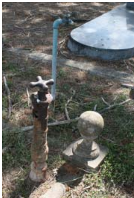
Figure 5-61. Two hose bibs within the Comal Cemetery. The one to the left may date from the original system installed ca. 1891. JMA, 2009.
