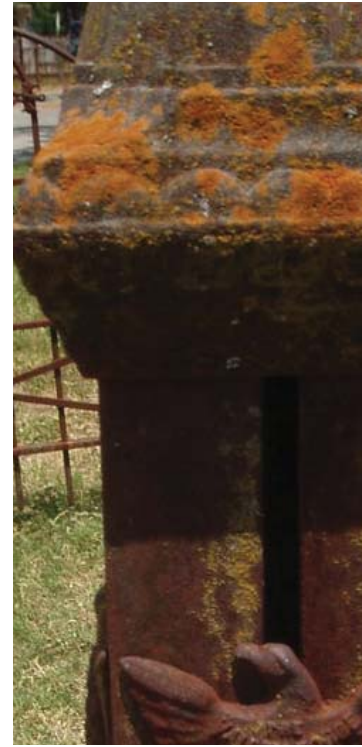
Figure 4-51. Rust bloom is evident on some elements. JMA, 2009.
