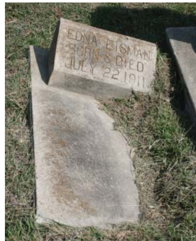
Figure 4-35. Concrete plot covering displaced by local soil subsidence. JMA, 2009.
