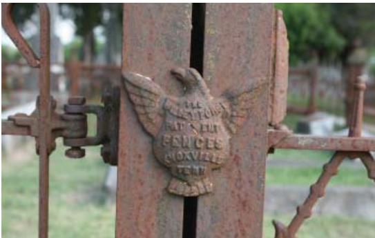
Figure 5-55. Faceplate exhibiting pitting and rusting. Protecting such features should be a high priority. JMA, 2009.
