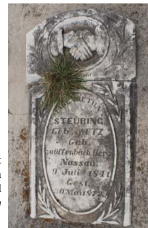
Figure 4-8. Encasement of this marker in concrete has hastened its deterioration. Cynthia J. Beeman, 2009.
