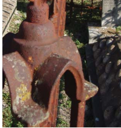
Figure 4-50. Pinhole damage and lichen are common on many elements. JMA, 2009.
