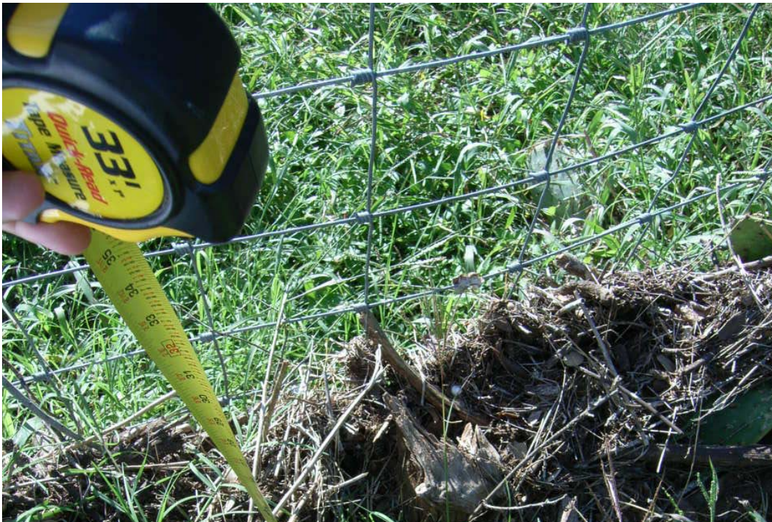
Buildup of debris that serves as obstruction to flow.
